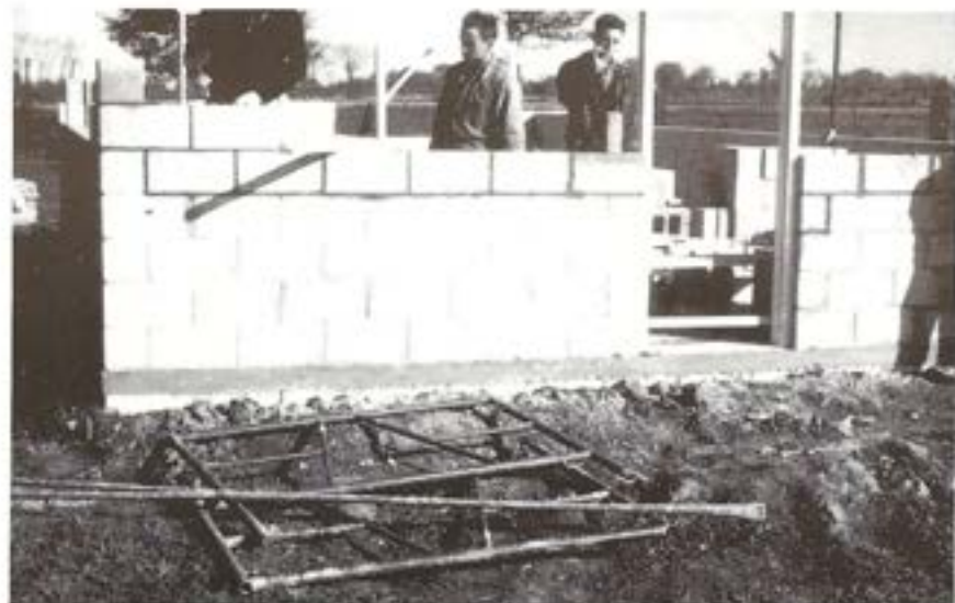
Building the Original Clubhouse. Many thanks to Harold Wakil of WAKIL CONSTRUCTION for a lot of labour and expertise donated. There was no heat or hydro in the Clubhouse yet, so the club continued to meet at Tait's farm.
